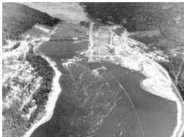
Figure 59. Aerial view of La Cave rapids during the construction of the bypass channel, 1949 (Hydro One Archives, Neg. No. 374)
