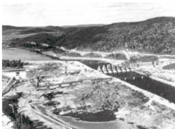
Figure 58. View of the substrate of La Cave Rapids during the construction of the Otto Holden Dam, 1950 (Hydro One Archives, Neg. No. E52-291).
